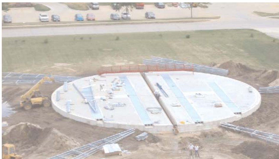
As evident from this photo, we'll be better able to "see" work progressing at our bin site as August begins. Roof sections are being assembled around the concrete foundation and dump pit excavation has been completed. Also visible at the bottom of the photo is the head section for the new leg that will be erected.
